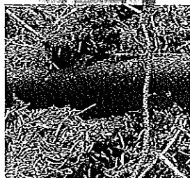
SeptiTech drip hose can be installed by hand under duff, pine needles or bark mulch.
